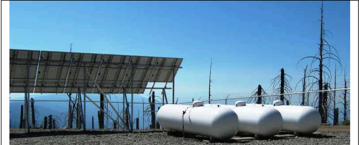
Above: Solar panels will charge batteries and propane tanks feed a backup generator to provide power to Pickett Peak cell tower. Note recent forest fire damage.
