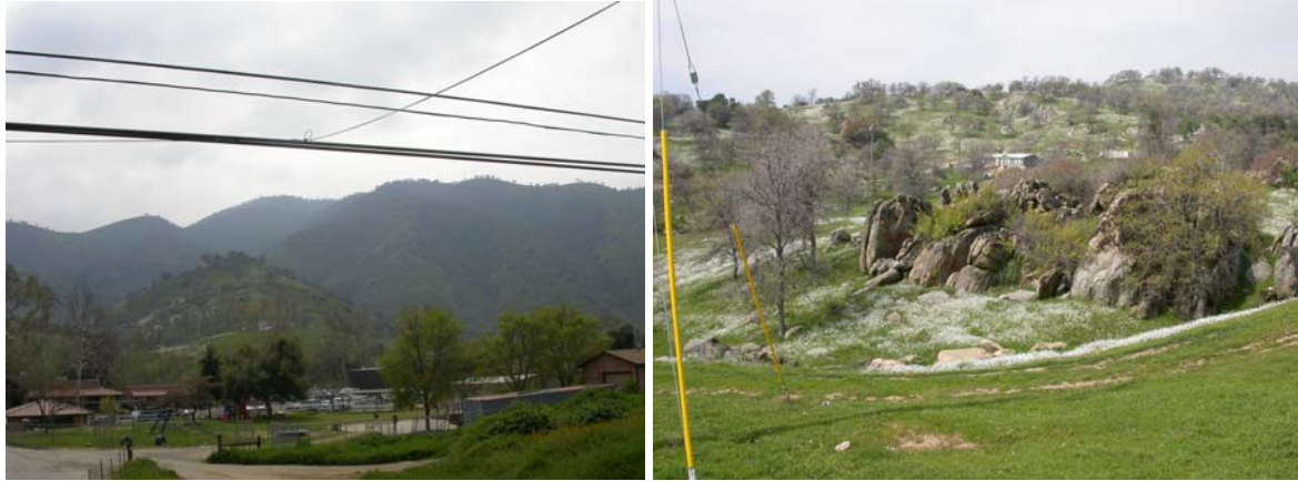
Left: Newly installed fiber optic with the Tule Tribe town center in distance. Right: New telecommunications plant atop Cow Mountain
