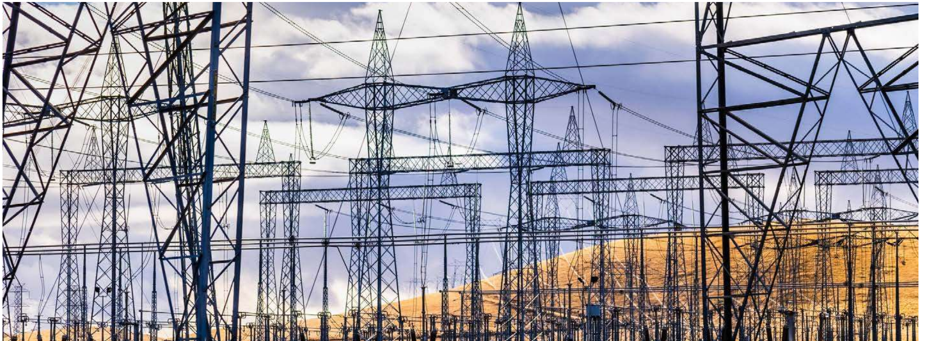
High-voltage electricity towers and power lines at a substation in Central California
