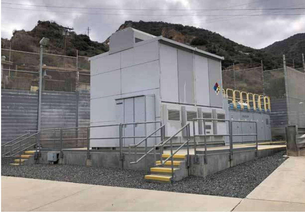
1MW battery storage facility on Catalina Island.
